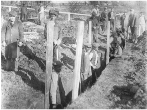
1930s – Workers employed by the Civil Works Administration dig trenches for sewer pipes on Snowden Avenue and Laclede Station Road.
